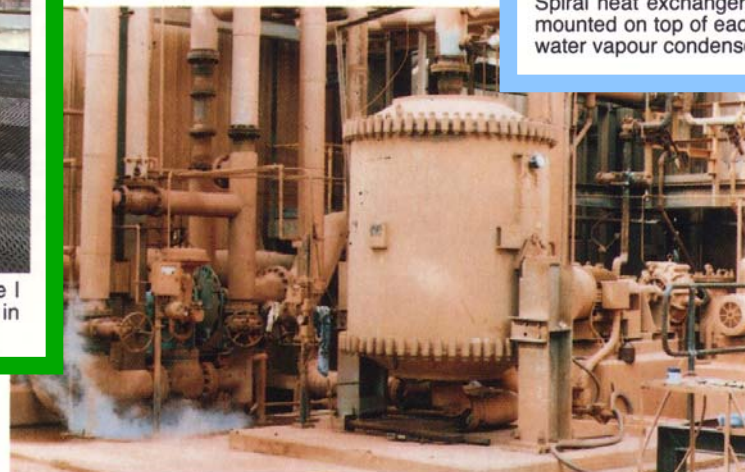
Queensland Alumina in Queensland, Australia, selected the spiral heat exchanger Type I for heating bauxite slurry.
