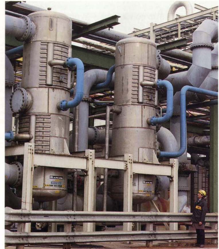
Spiral heat exchanger units consisting of two spiral heat exchangers Type II mounted on top of each other are used by ICI in Billingham, the UK, as partial water vapour condensers in the ammonia plant.
