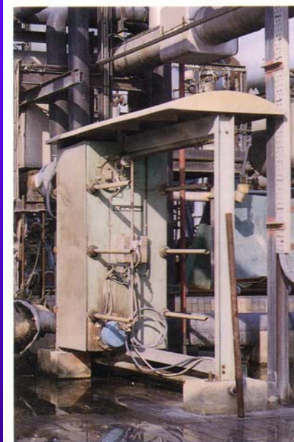
Tioxide France in Calais, France, chose plate heat exchangers with welded plate pairs and anodic protection to cool concentrated 100°C (212°F) sulphuric acid.
