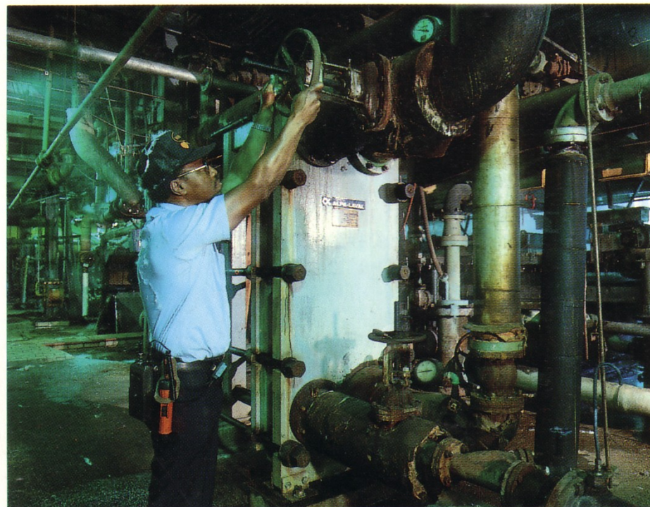
At Courtaulds North America in Axis, Alabama, plate heat exchangers maintain the correct temperature of the washing baths in the viscose plant.
