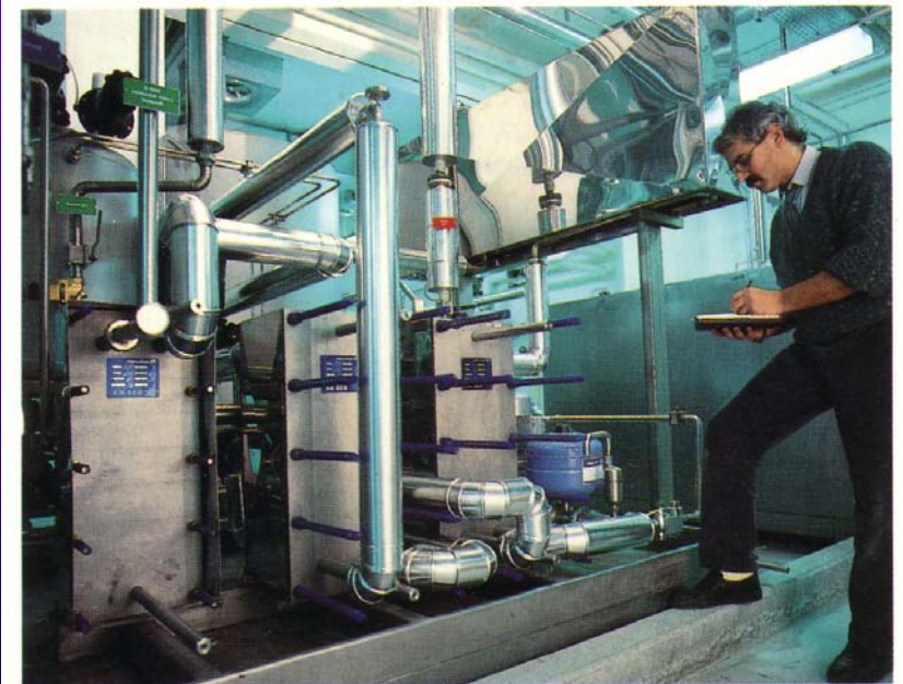
At Sandoz AG in Basel, Switzerland, these three Double-wall plate heat exchangers in the biotechnology pilot plant heat and cool toxic waste products using city water.
