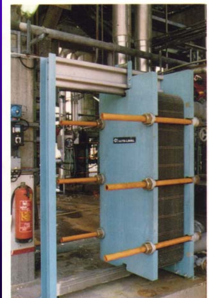
At DSM, Beek, the Netherlands, plate heat exchangers from Alfa-Laval serve as reactor jacket water coolers in the polypropylene plant.
