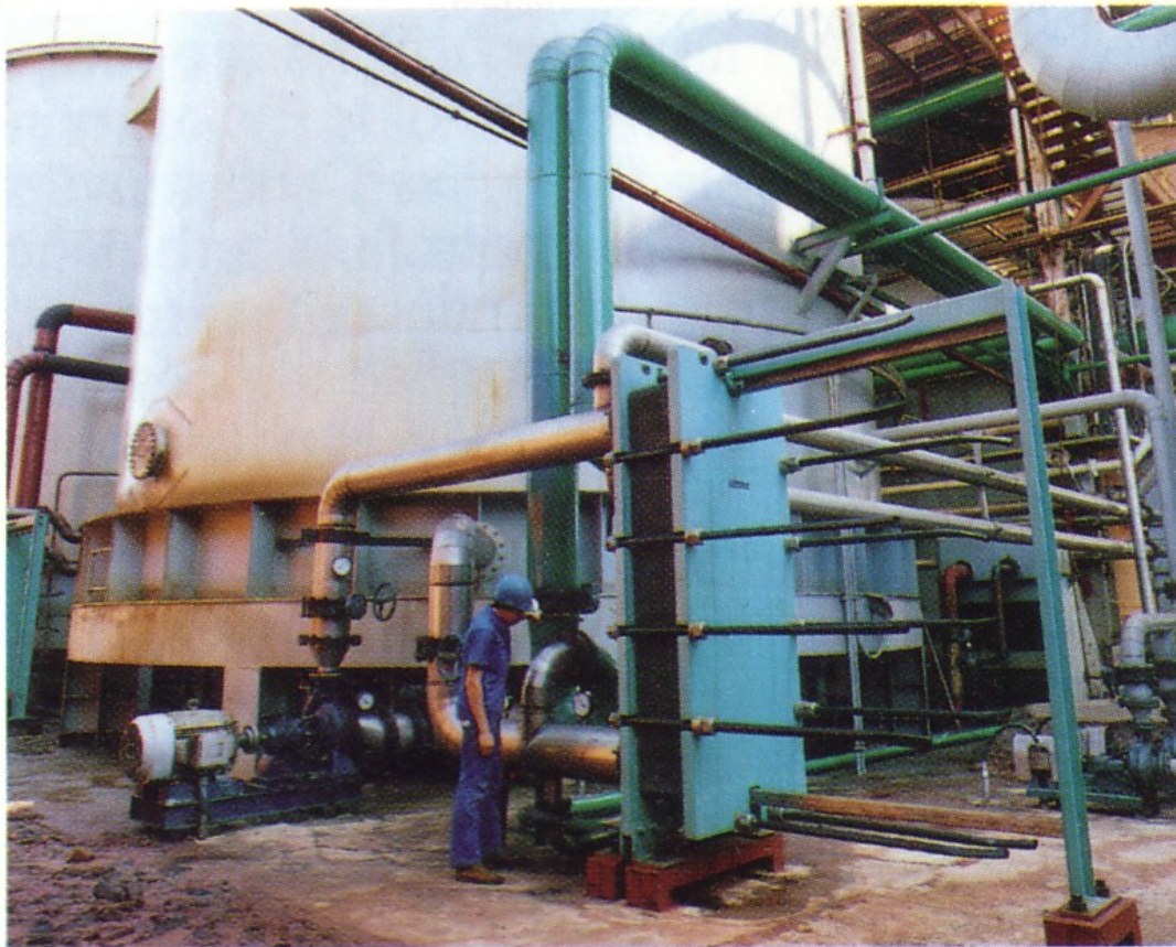
A plate heat exchanger installed as a fermenter cooler at the Usina de Serra distillery in São Paulo, Brazil.
