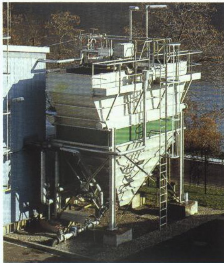
Figure 317. Metal Sédipac. Facility in Rheinfelden, Germany.
