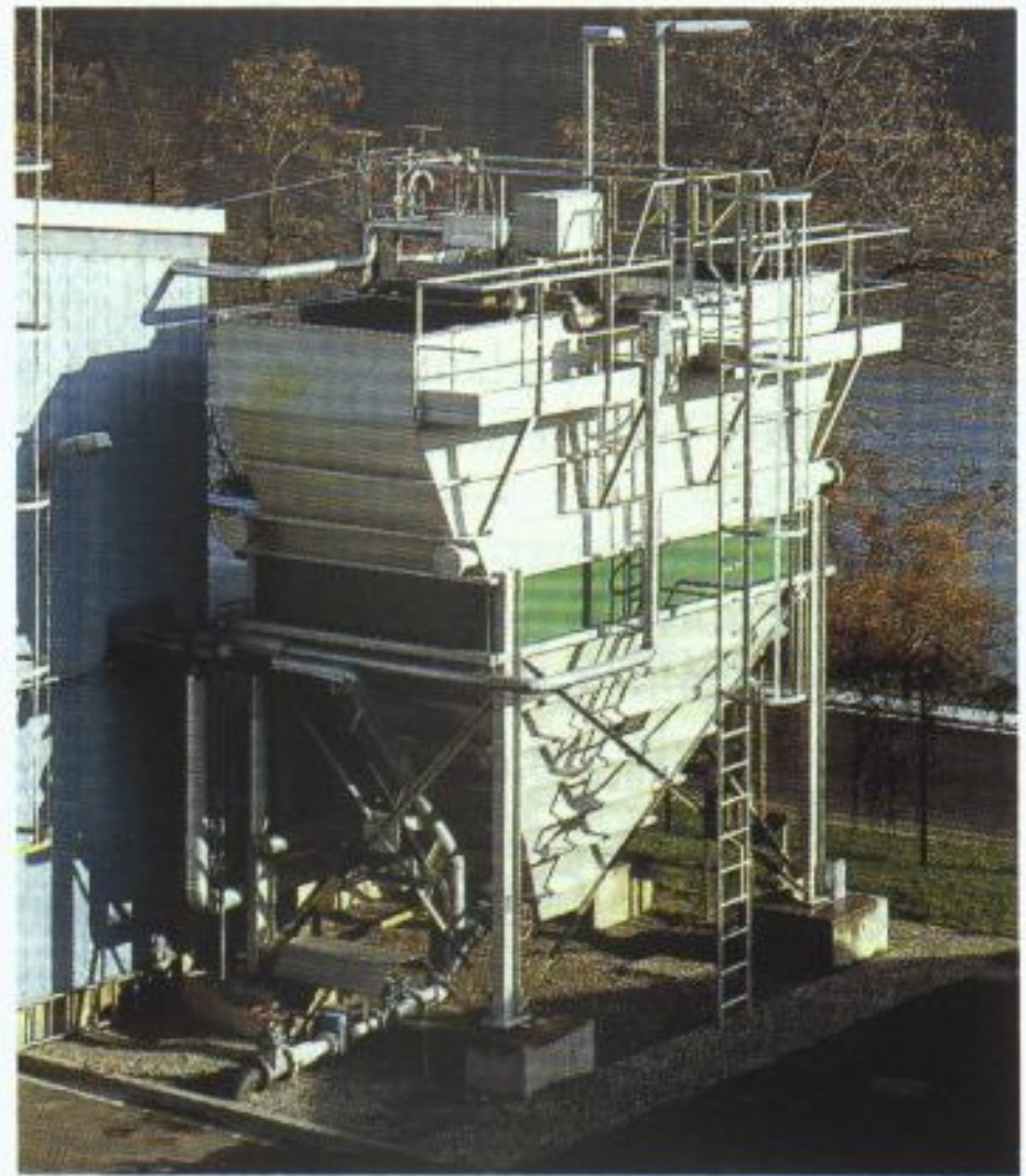
Figure 317. Metal Sédipac. Facility in Rheinfelden, Germany.
